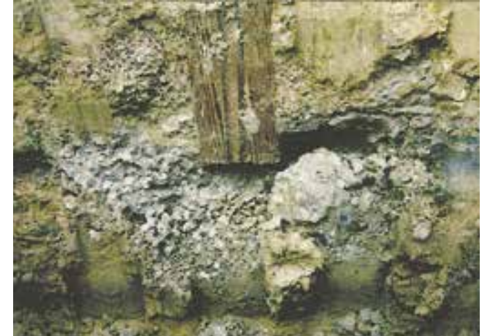
Example of powder concrete bag foundation (Not Recommended)
